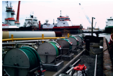
3" Couplings on hose reels for loading supply vessels with various chemicals
