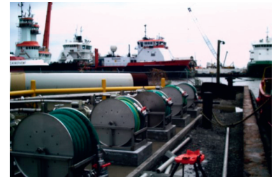
In blending plants for a clean working environment. Selectivity options available to avoid cross-contamination.
